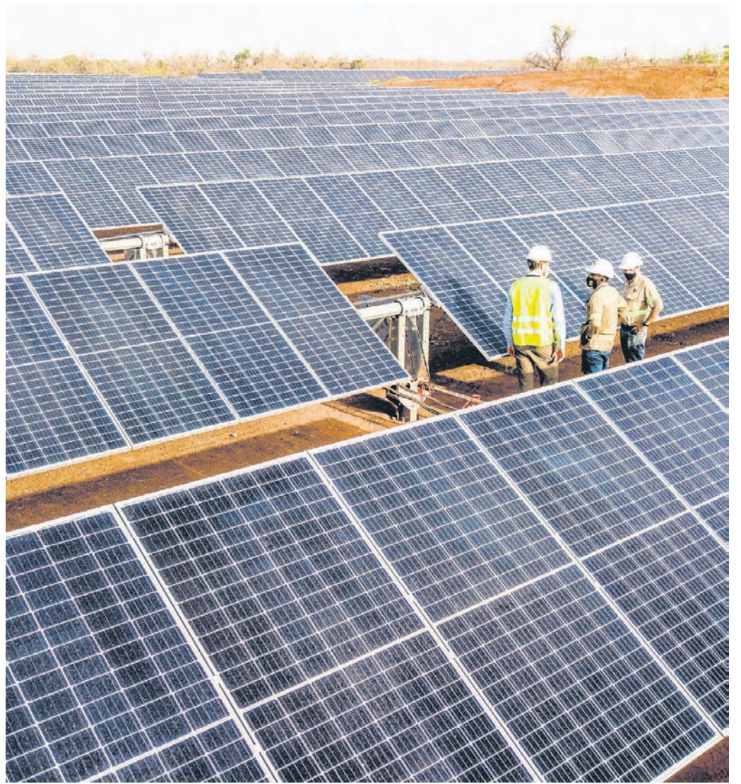
A solar installation at B2Gold's operation in Fekola, Mali, is enabling the organization to significantly reduce its reliance on fossil fuels. SUPPLIED
